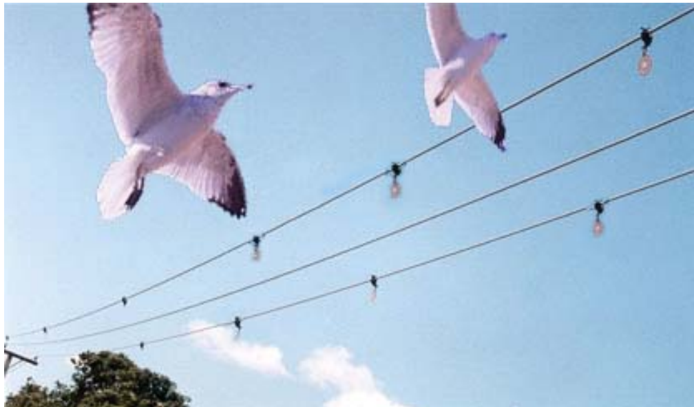
Figure 3: Flight diverters installed on parallel lines.
