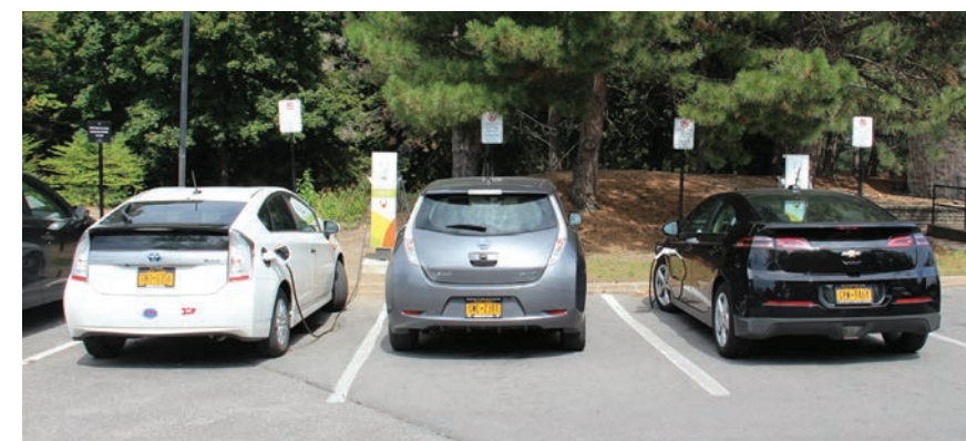
Two electric vehicle charging stations were installed in the Facilities parking lot. The chargers can service up to four vehicles at a time, and work for both electric-only vehicles and plug-in hybrids.
